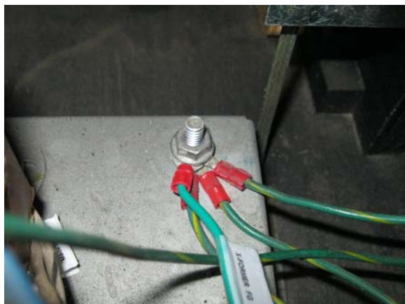
Figure 49 - Transformer Chassis Plate Grounds
